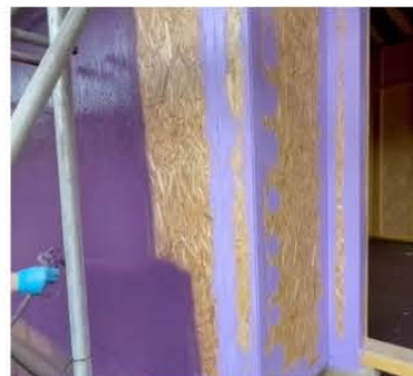
Passive Purple External brush applied to timber frame wall connection before the application of Passive Purple External.
